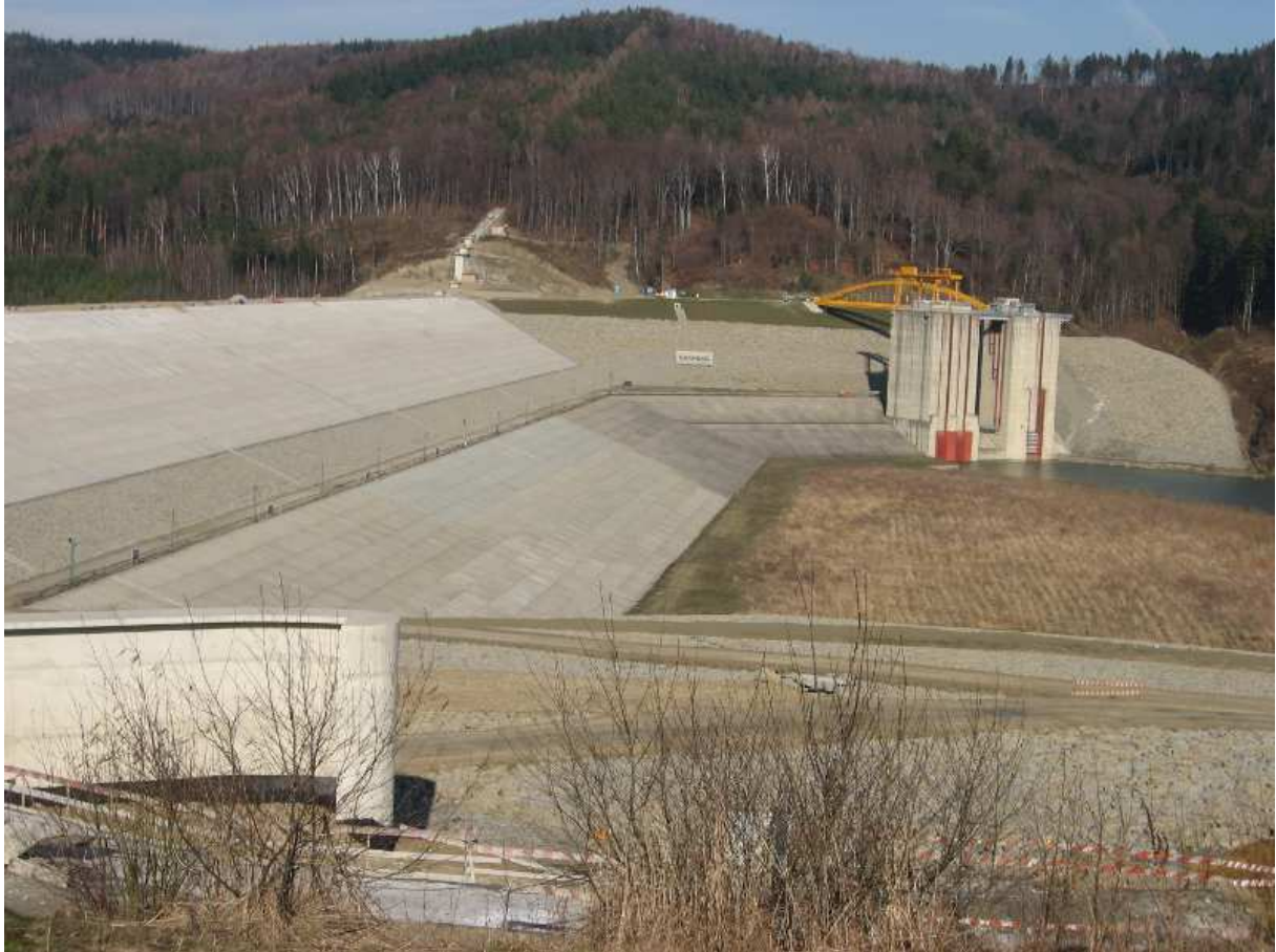
Fig.41 An earth dam in Świnna Poręba, Poland. Image taken before the reservoir has been filled with water. You can see the protection of the inner side of the dam with concrete layers and rocks. Author: Gambitek. Source: Wikipedia [W12].
